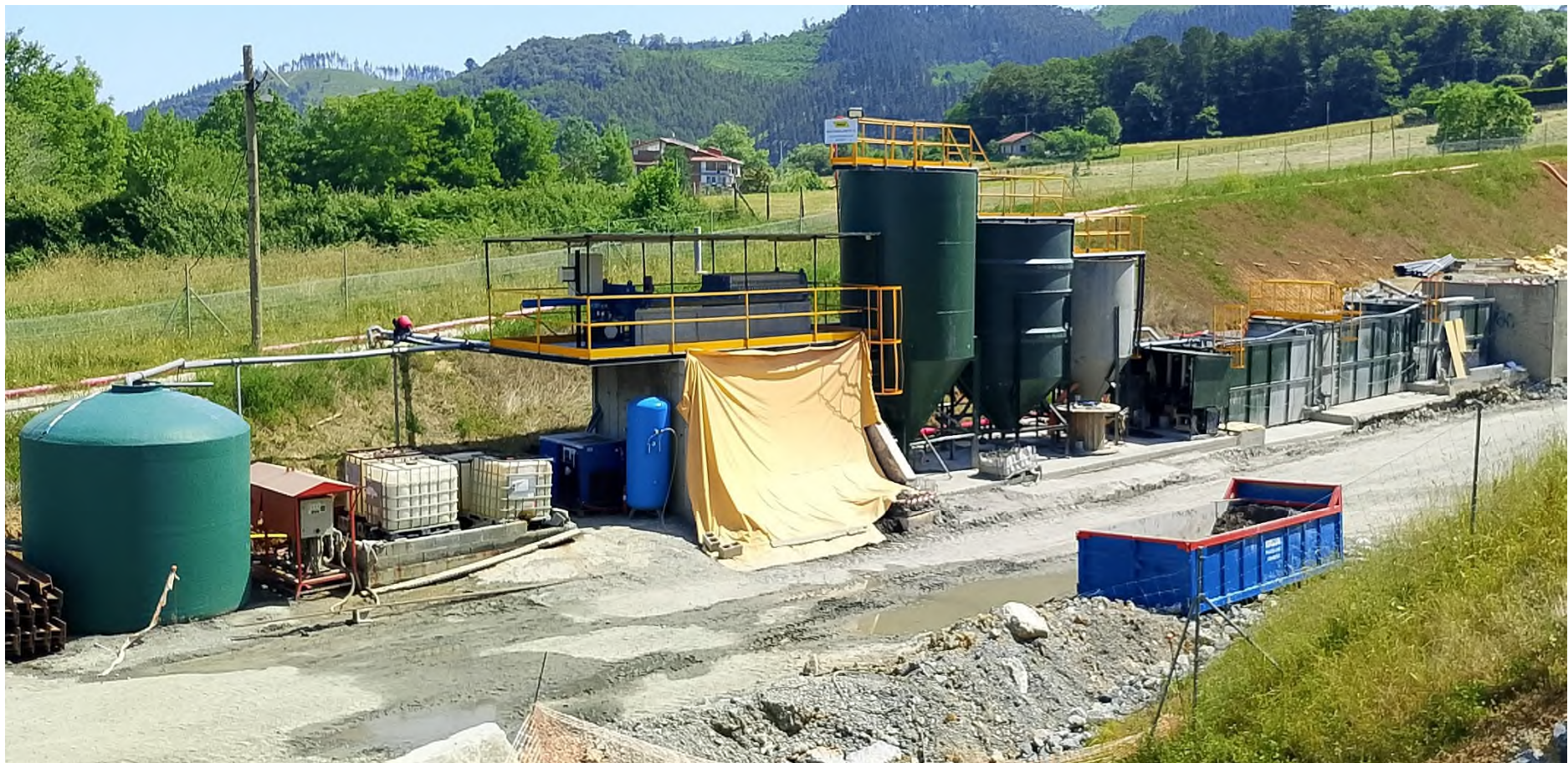
DEPURADORA EMBOQUILLE MARKINA
